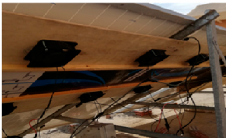
Figure 6: PV Air cooling Layout
